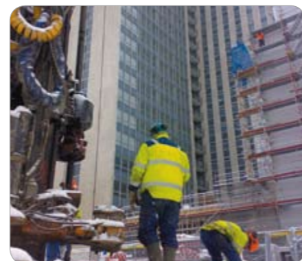
Rosenlundsterrasen, Stockholm – Sweden Foundation work in a sensitive area close to a highway tunnel.
