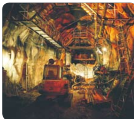
Hallandsåsen – Sweden Installation of 100 meter long freeze pipes under difficult ground conditions.
