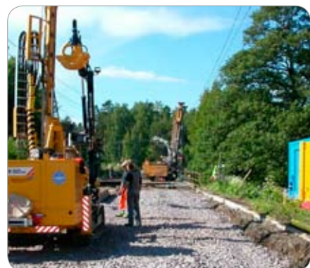
Fagersta – Sweden Reinforcement of foundations for a railway bridge, close to a drinking water supply area.
