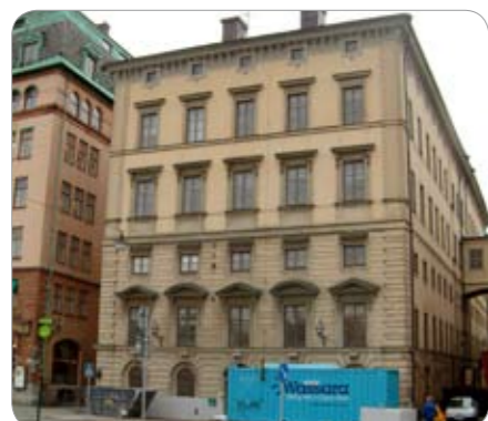
Bancohuset, Stockholm – Sweden Reinforcement of the unique Banco building in Old Town, Stockholm.
