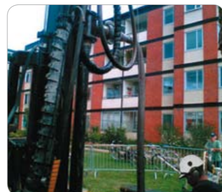
Tunahus, Lund – Sweden Geothermal drilling to reduce heating costs for over 200 apartments.
